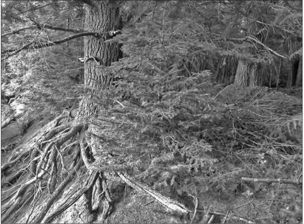
Figure 5. River bank erosion (left) within 5 m of foundation mound (right). R. MacKay collection.
