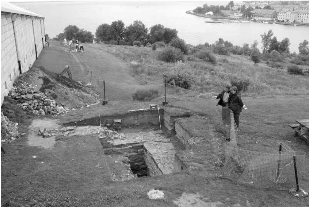
Figure 4. Excavations on the southwest corner of the 1820 Officers' Barracks, facing south. (Photo 131H653E by H. Cary).
